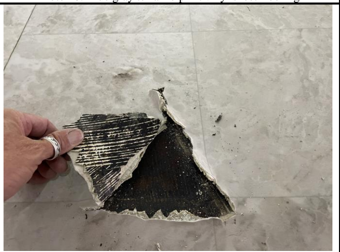
Photo 12: ACM flooring under sheet vinyl
