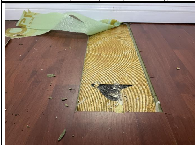
Photo 11: ACM flooring under laminate
